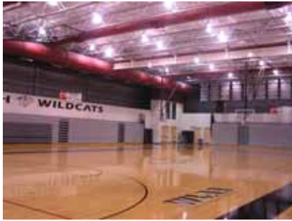
Existing Gymnasium Lighting
