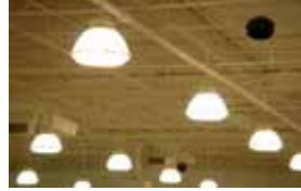
Induction Lighting 60% more efficient
